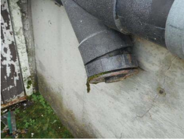
The plastic roof drain was broken.
