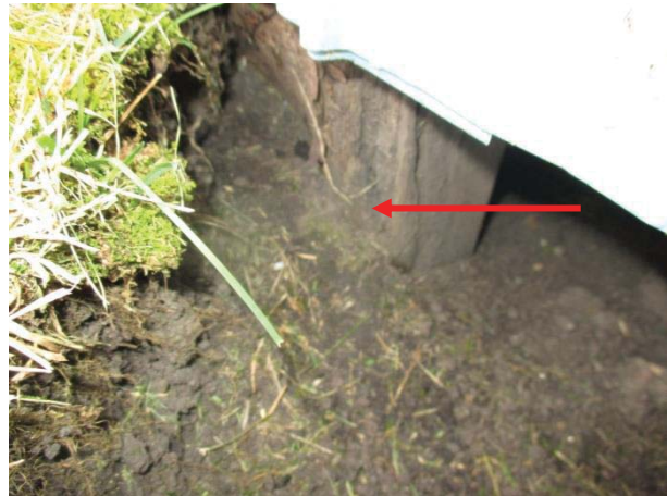
The wooden posts used to support the skirting around the portables were rotten.
