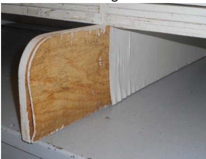
Water damage from past water leakage through roof.
