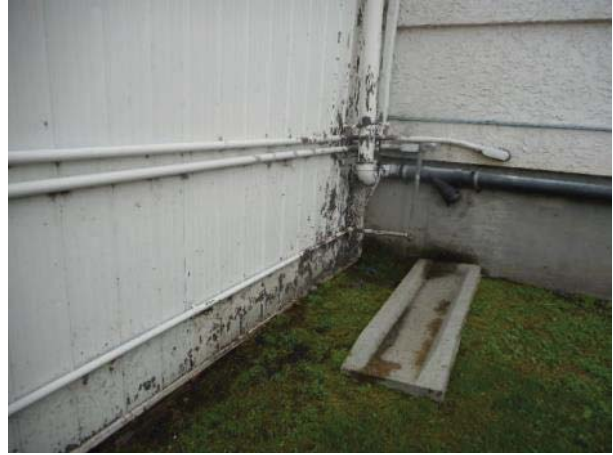
Water inundation occurring at the corner where FS-109 is joined to the gymnasium.
