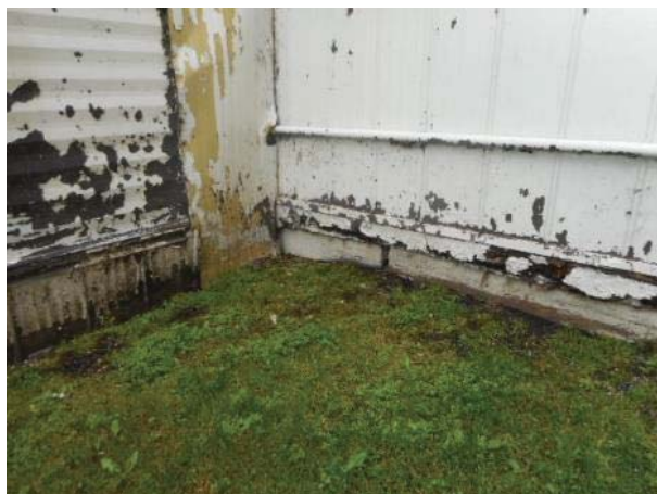
A close up of the corner where FS-109 joins the library portable.
