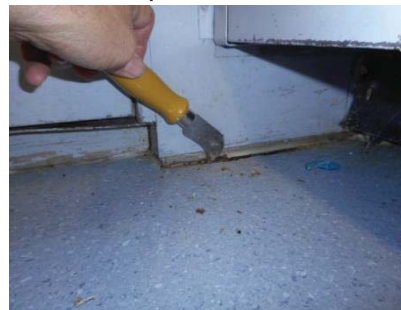
Floor underneath the Palm-Air was rotten.
