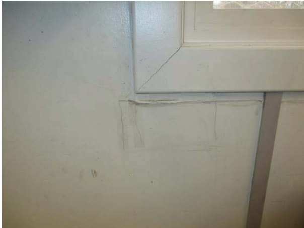
Localized water damage was noticed under the window on the east wall. The drywall was dry <10% (acceptable),
