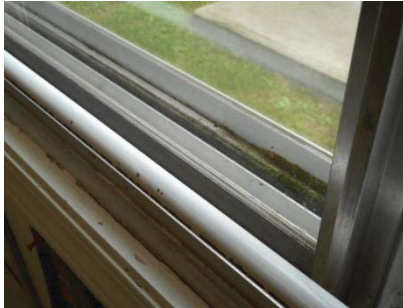
Moss growth in the window tracks.
