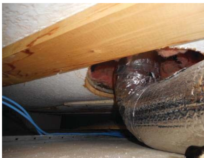
Mould growth above the old ceiling by the roof drain, in the northwest corner Stachybotrys sp. Sample #4437.02
