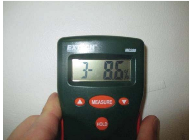
Moisture readings around the east window and all accessible walls were <10% moisture, acceptable.
