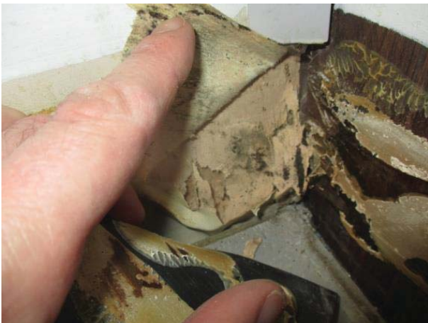
The rubber baseboard was removed from the northeast corner of the classroom. Mould growth was identified on the drywall paper Chaetomium sp. , Sample #2
