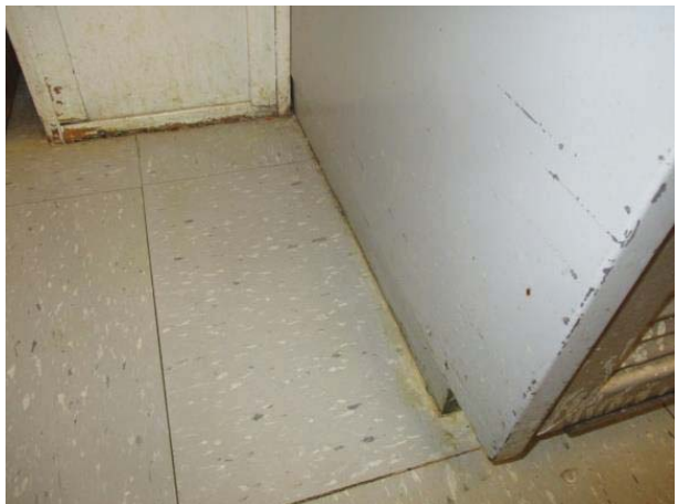
Water staining was noticed on the floor tiles and along the bottom of the air intake cabinetry.
