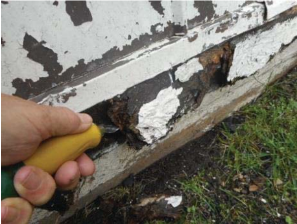
The north wall of FS-109 was rotten.
