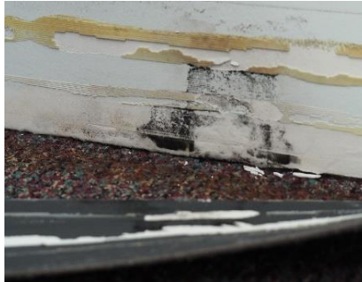
Photo #10: Sample 4468.04 Stachybotrys sp. On the front face of the drywall.
