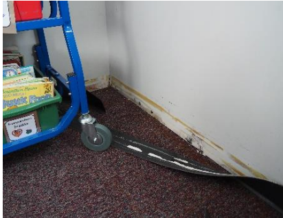
Photo #9: Northeast corner with baseboard peeled back.
