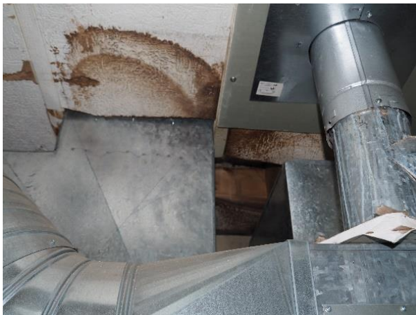
Photo # 12: Water damaged original ceiling in the mechanical room of FS-115.
