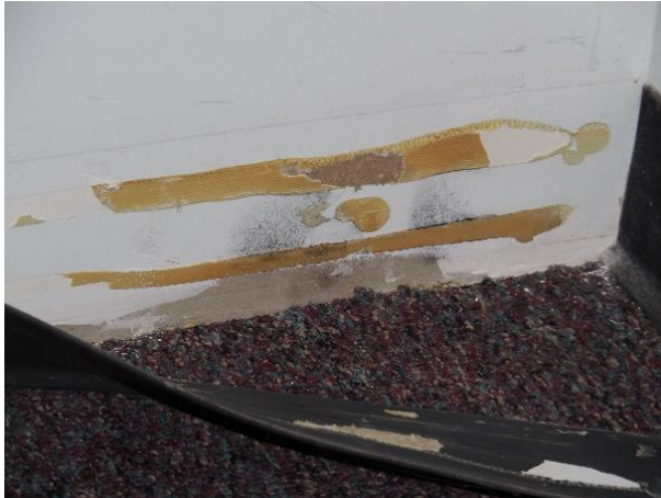
Photo # 13: Mould growth behind the baseboards on the west wall under the window adjacent to the air return grille.
