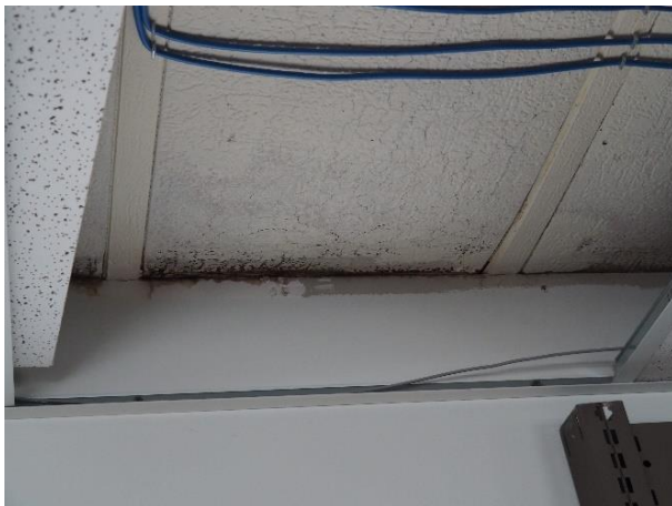
Photo #4: Above the new suspended ceiling tiles is the original cellulose ceiling with water staining.
