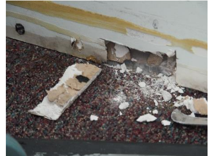
Photo #11: Chaetomium sp. On the reverse side of the drywall.
