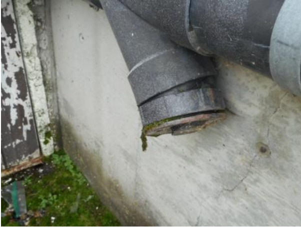
The plastic roof drain was broken.
