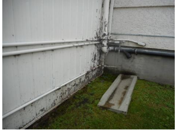
Water inundation occurring at the corner where FS-109 is joined to the gymnasium.
