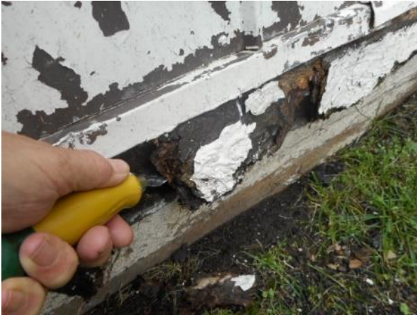
The north wall of FS-109 was rotten.
