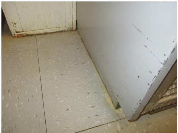
Water staining was noticed on the floor tiles and along the bottom of the air intake cabinetry.
