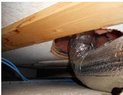
Mould growth above the old ceiling by the roof drain, in the northwest corner Stachybotrys sp. Sample #4437.02
