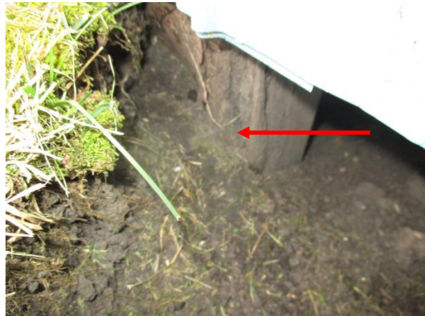
The wooden posts used to support the skirting around the portables were rotten.
