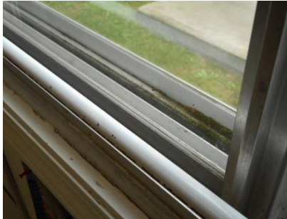
Moss growth in the window tracks.
