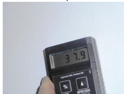
Moisture reading on the east wall by the furnace, above rubber baseboards.
