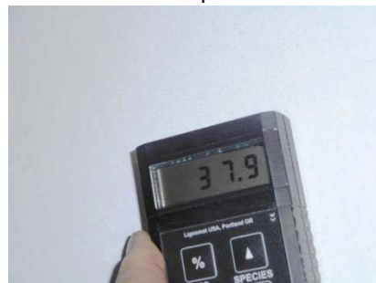
Moisture reading on the east wall by the furnace, above rubber baseboards.
