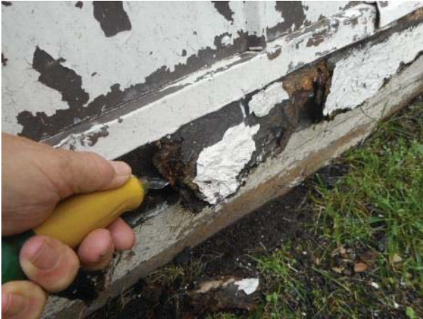
The north wall of FS-109 was rotten.
