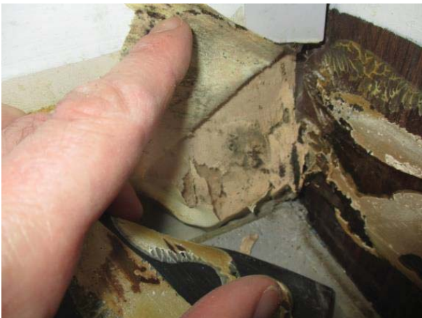
The rubber baseboard was removed from the northeast corner of the classroom. Mould growth was identified on the drywall paper Chaetomium sp. , Sample #2
