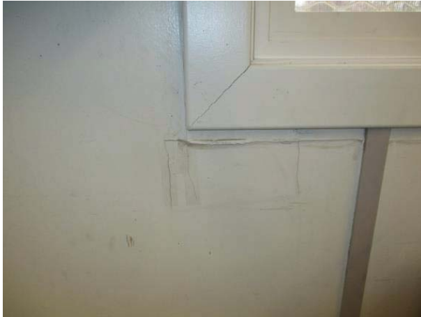
Localized water damage was noticed under the window on the east wall. The drywall was dry <10% (acceptable),
