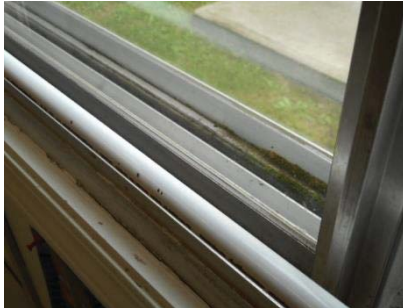
Moss growth in the window tracks.
