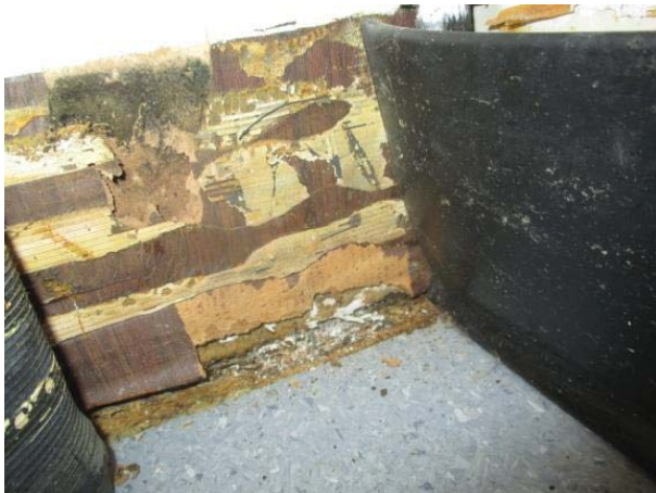
The rubber baseboard was removed from the southeast corner of the classroom.
