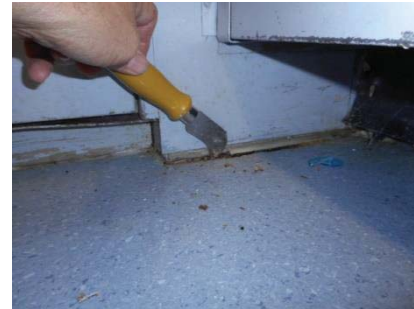
Floor underneath the Palm-Air was rotten.
