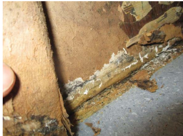
Mould growth was evident on drywall paper Stachybotrys sp. Sample #1.
