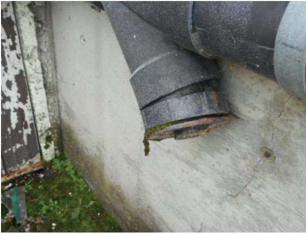
The plastic roof drain was broken.
